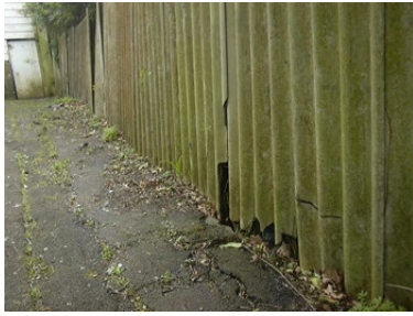
Asbestos Fence Panels
