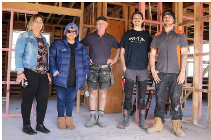
Work is underway at the first home to be repaired through the Wairoa Mayoral Relief Fund. Pictured from left is Deputy Mayor Denise Eaglesome Karkare, homeowner Wiki Hauraki, Wayne Jacobs of WJ Construction in the Waikato who has donated two weeks of time, Kohi Poharama who is offering voluntary work on the rebuild and Hugh Eaglesome-Karekare of Savage Electrical Solutions.
