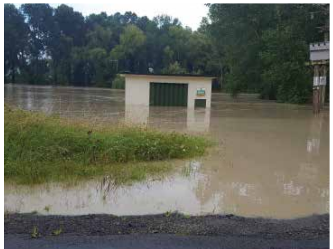
Picture of Wairoa water intake during Cyclone Gabrielle. This caused major issues in terms of water supply and damage to the water treatment infrastructure.
