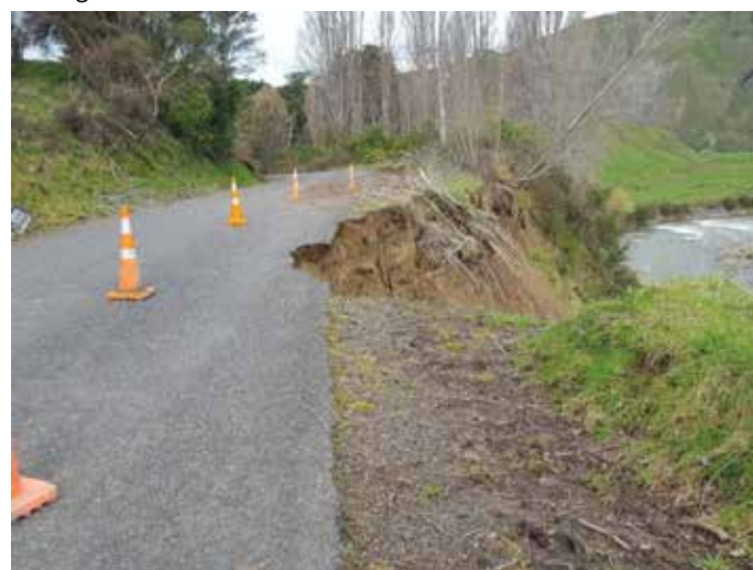
Ruakituri Road Dropout
